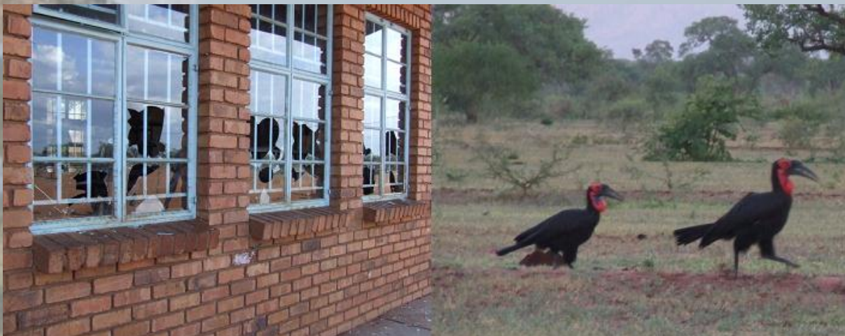
Windows broken by ground hornbills
